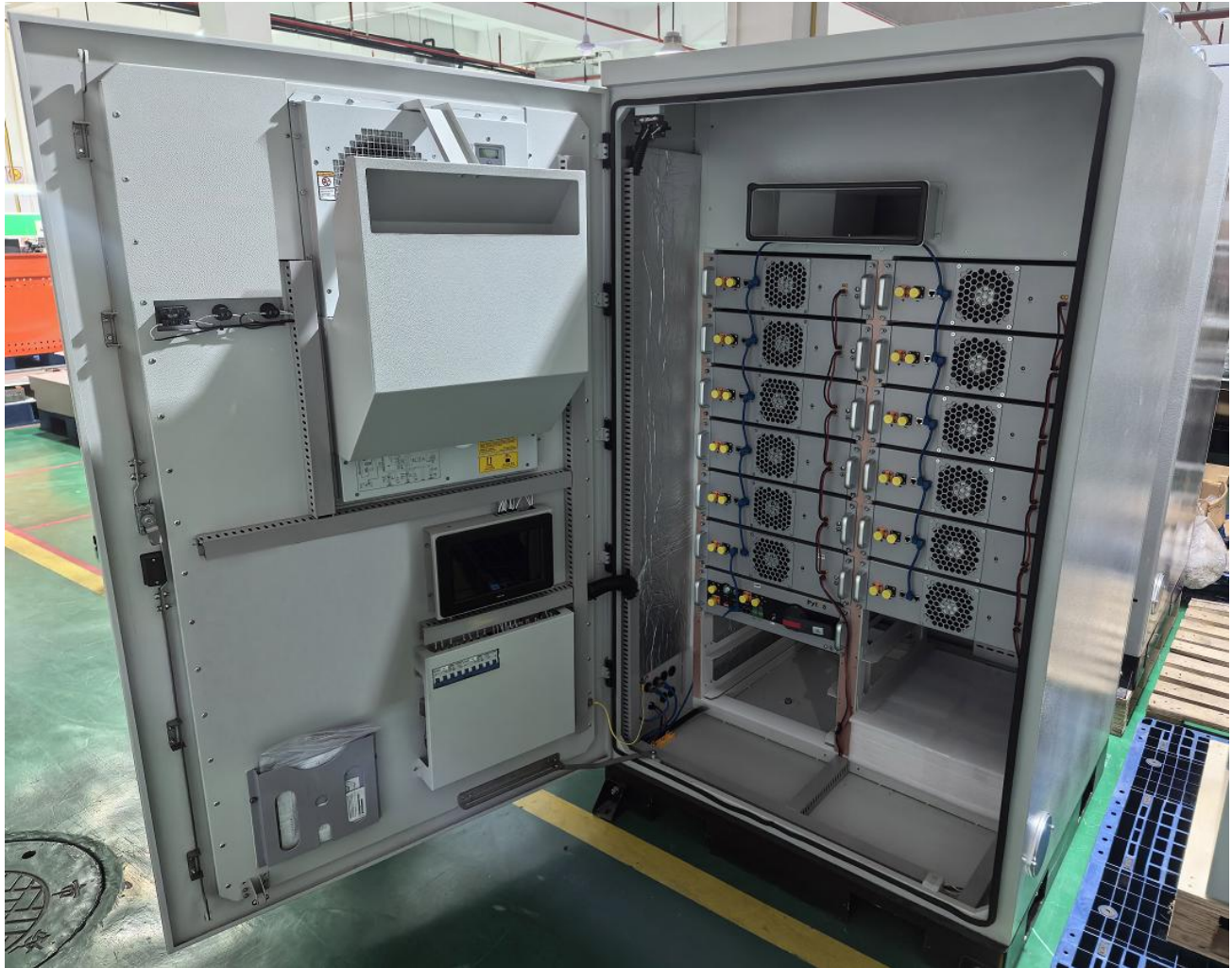
Photo 4: Internal View of DC Energy Storage System (representative model HV48100 SE Lite 1P12S ESS)
