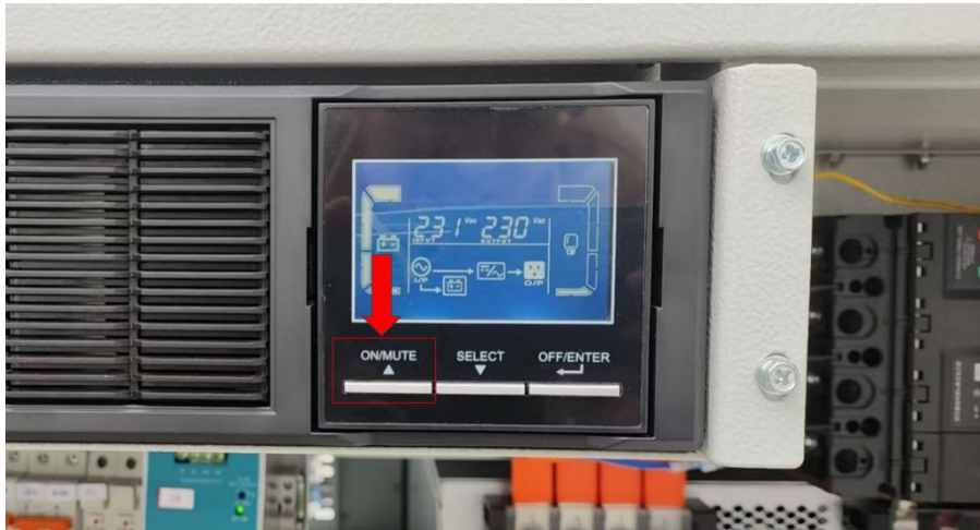
Figure 6.5 Turn on the UPS
